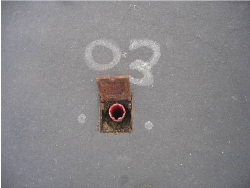
Plate 22 Scarborough South Cliff H6 (AA03)
